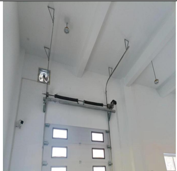
防爆监控、换气扇
